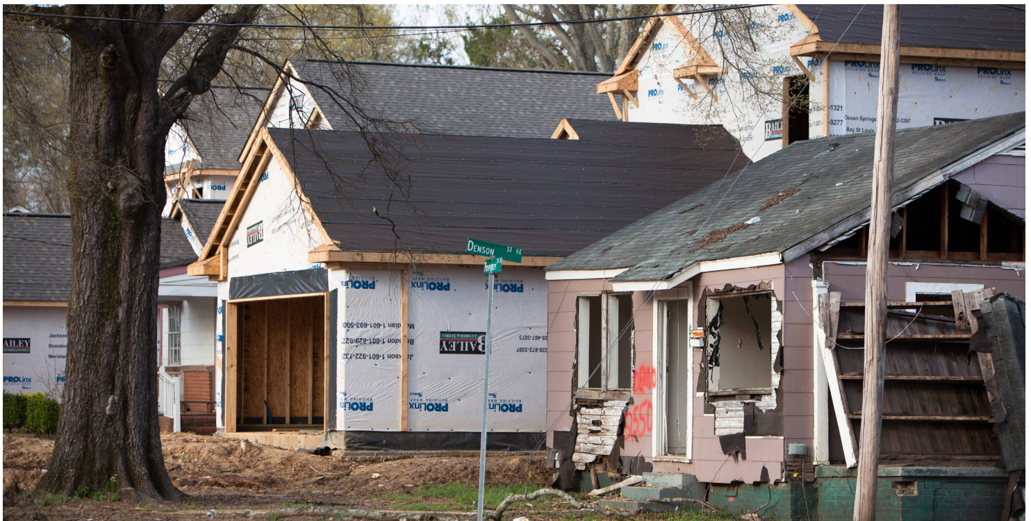
Construction of houses in the area of the Jackson Medical Mall in Jackson, MS.
